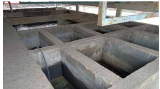
Cables Division's water recirculating system.
